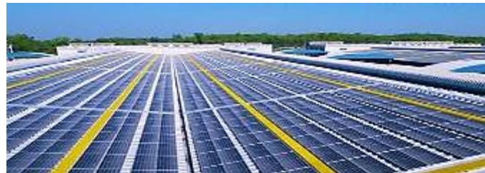
[Rooftop Solar Panel in KEPZ]
