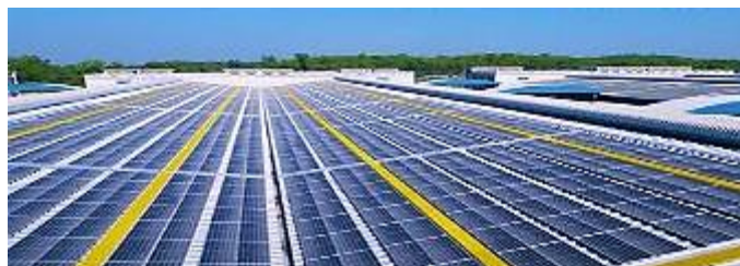
[Rooftop Solar Panel in KEPZ]
